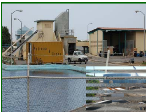
Picture a wastewater treatment plant
